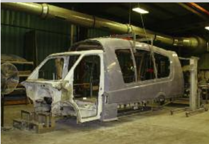
Here, the body panels of the Mauck2 are bonded to the frame. The use of a jig chassis ensures proper fit and alignment between the body and chassis.
