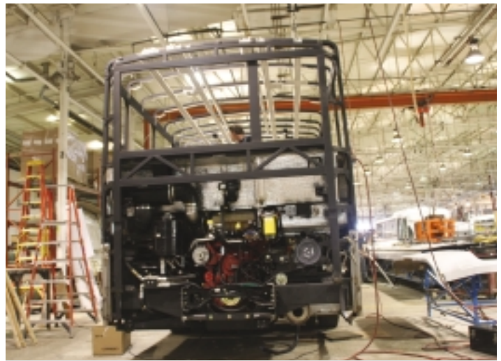
Further down the GCA assembly line at Imlay City, we see the web frame body structure of the 3035RE taking shape. GCA also builds a cutaway type bus for ABC using an FCCC chassis. NBT.
