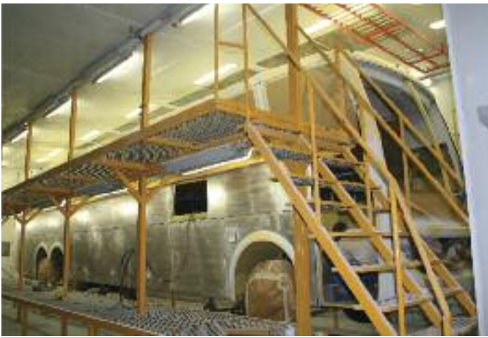
A CAIO bus headed for the United States is shown in one of several paint booths.
