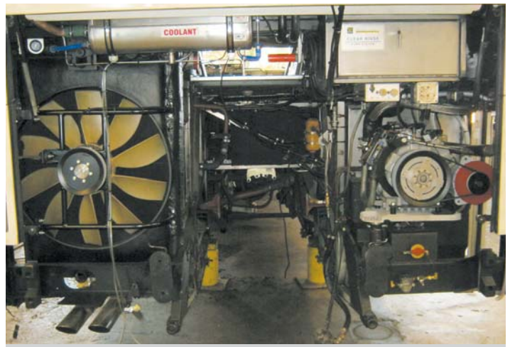
This photo shows a C2045 partially through the refurbishing process. Much of the engine compartment has been updated with new components. Next, a newly rebuilt engine will be installed to complete the process.
