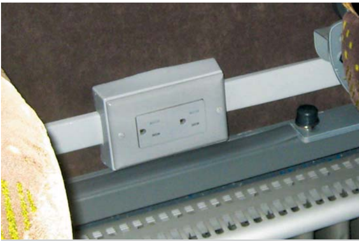
Since more and more passengers are walking on board your coach with laptop computers, installing 110-volt outlets and WiFi during the refurbishing process is an obvious option.
