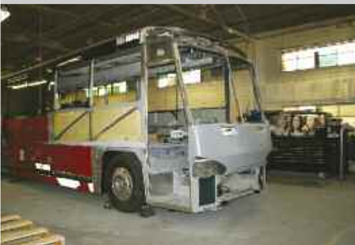
Collision repair has become the major activity at Loudonville. This particular coach suffered a head-on collision and is being rebuilt from the front back two passenger windows.
